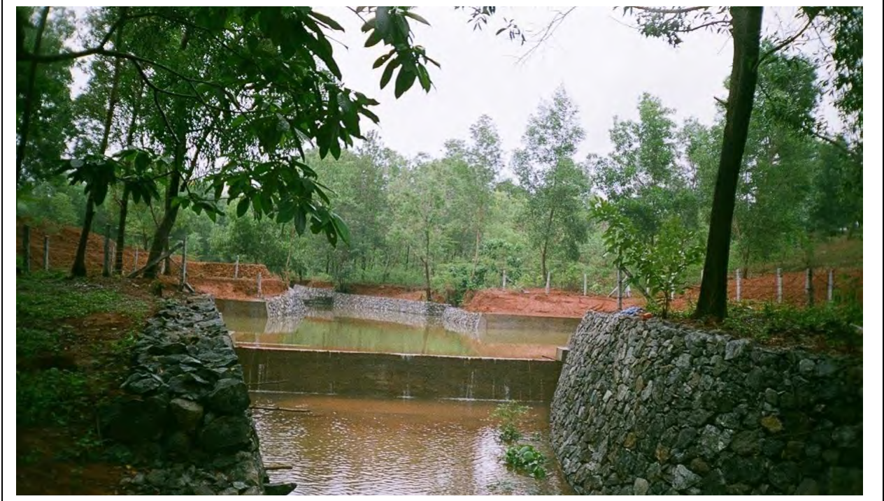
Check Dam with Bund protection work at Govt College, Manjeswar, Kasargod
