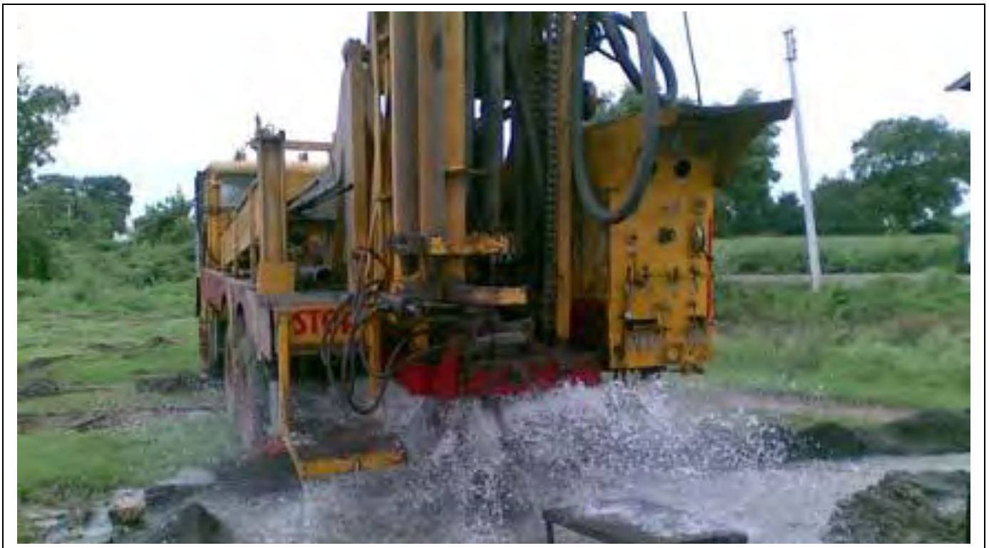
High Yielding Well at Satrasen EW, Chopda Taluka, Jalgaon District.
