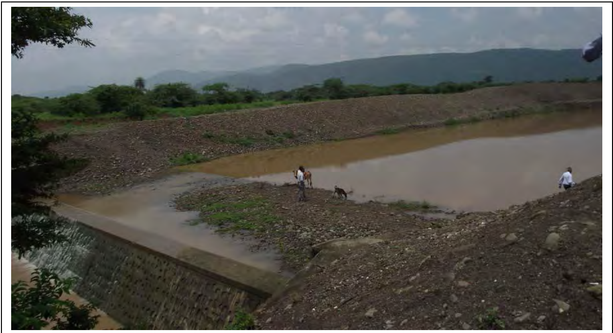
Inspection by Technical Committee of at Nala Deepening on Shirpur Pattern at Pala, Warud Taluka, Amravati District.
